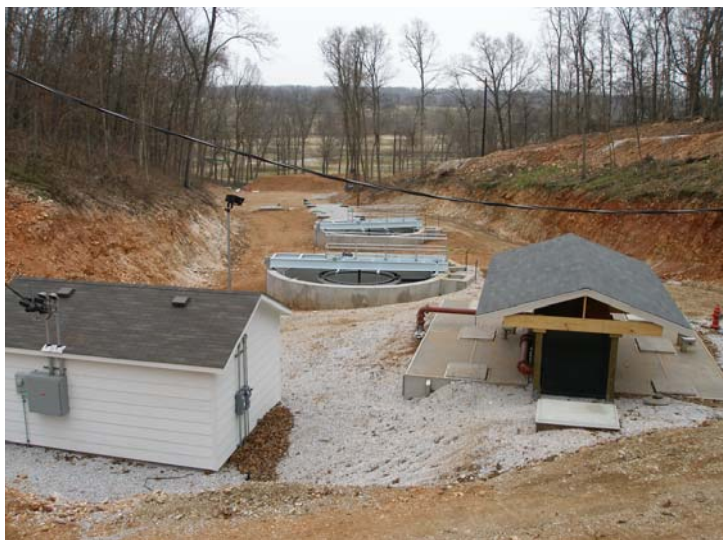
A 320,000 gpd Lotus-ActiveCell WWTP for 1,250 homes and A commercial downtown area. Effluent is reused for irrigation.
